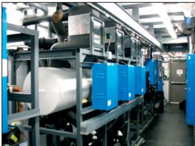
Figure 2. CO 2 Secondary Coolant System Installation at Food Lion
