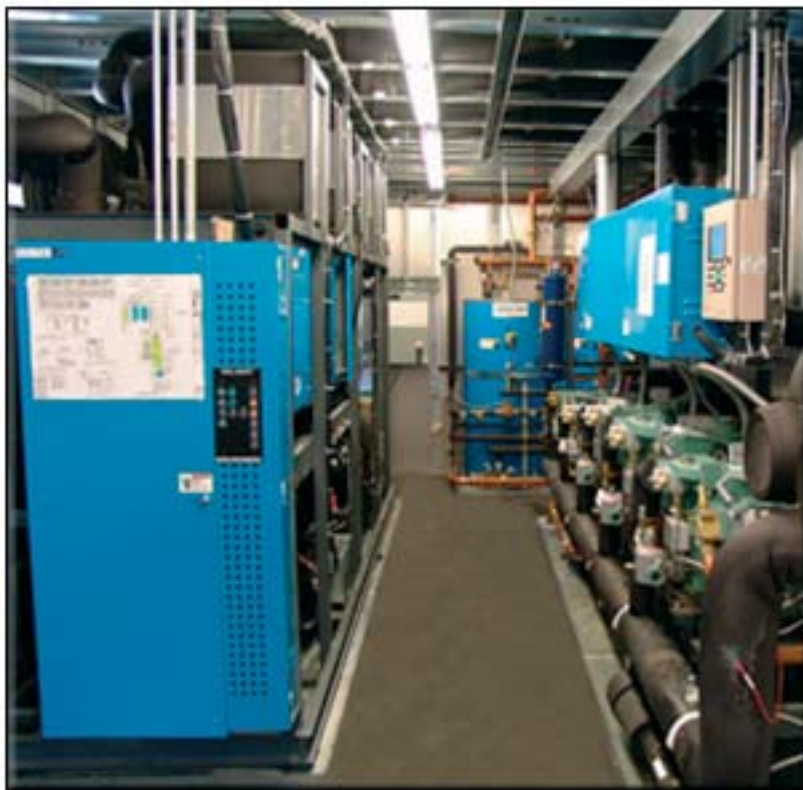
Figure 1. CO 2 Secondary Installation for a Wal-Mart Warehouse-Style Store
