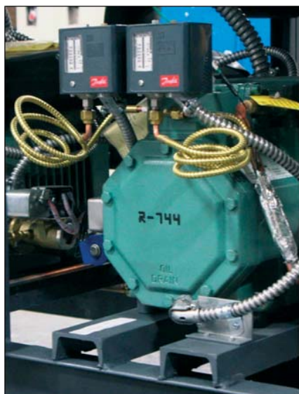
Figure 4. CO 2 Cascade Compressor
